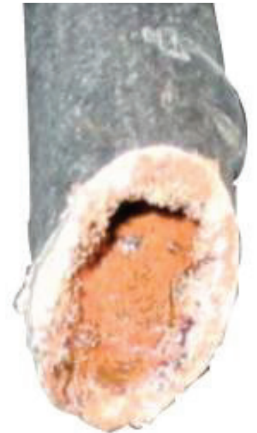
Lead service line
